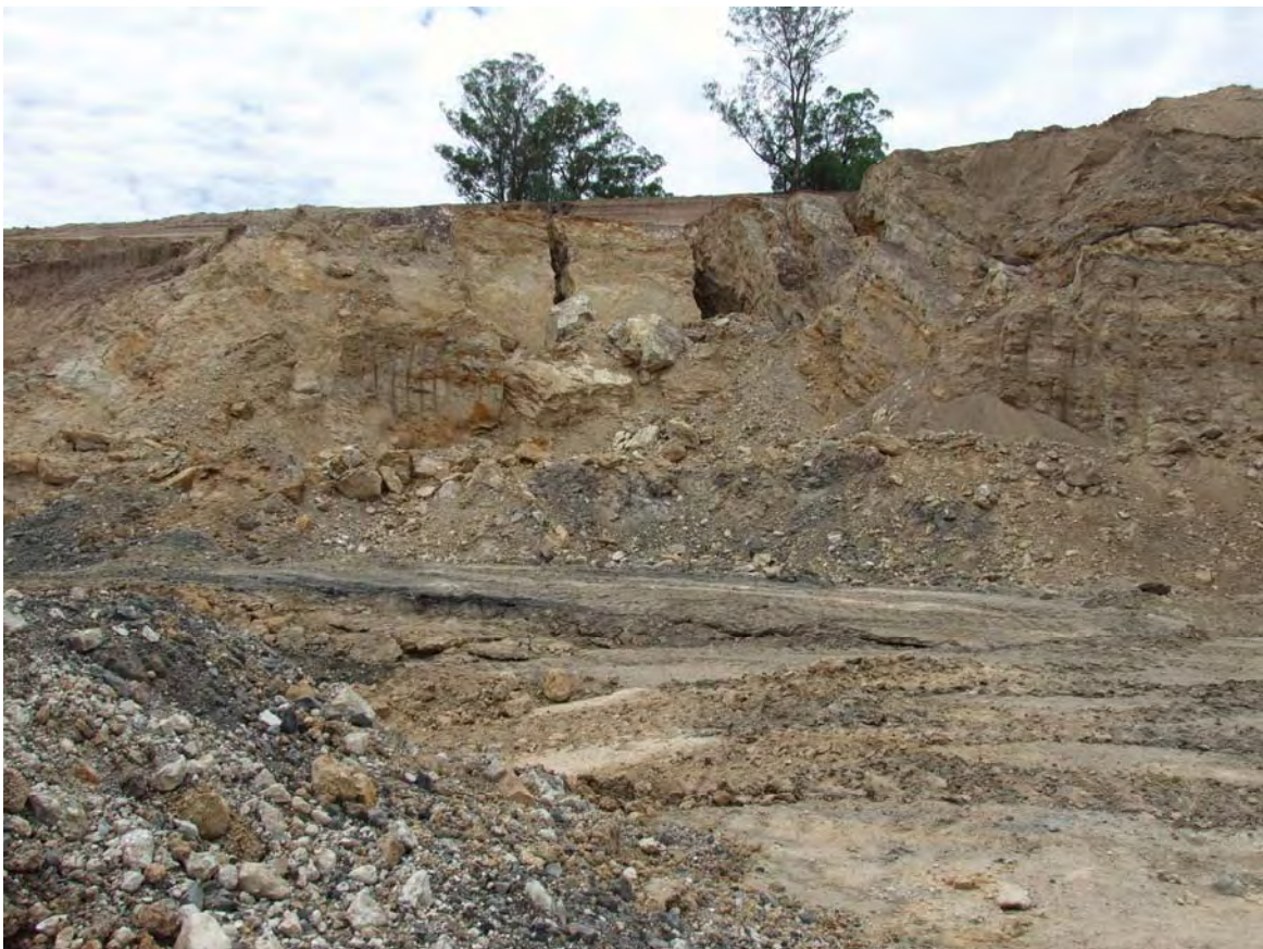
Figure 2: Sidewall of pit showing slumped strata in front of fault
